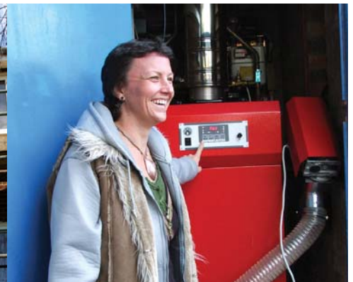
Gail Bamford and the Italian-made bio-mass boiler.
