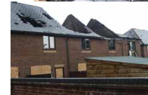
It will be months before these Hazel Housing Co-operative properties are habitable again
